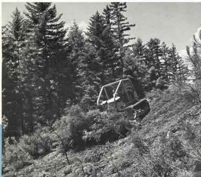
Tractor clearing the way for logging road. Logging companies find the Brush Grubber an inexpensive and economical tool that performs many tasks.
