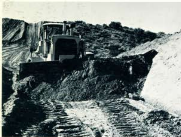
Sloper Blade on the move cutting clean slope. Note full blade load. Sloper attachment aligns with top of dozer blade in all positions eliminating spill back. Some slopes on this highway job were cut with just two passes.
