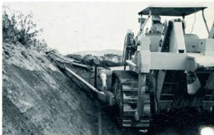
Beautiful slopes like this are cut in just minutes, a real time saver. Note the CLEAN SLOPE TOE, no material left behind for tractor crawler tilt, a prime requisite for accurate sloping operations.
